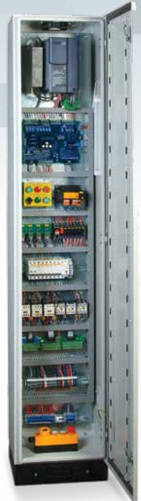
MRL ASANSÖR KUMANDA PANOSU MRL LIFT CONTROL PANEL
