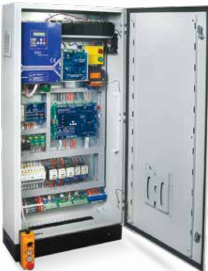
HİDROLİK ASANSÖR KUMANDA PANOSU HYDRAULIC LIFT CONTROL PANEL
