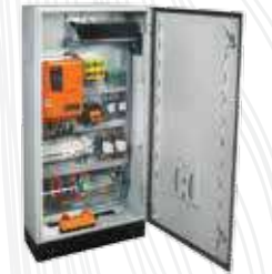
Pano Control panel
